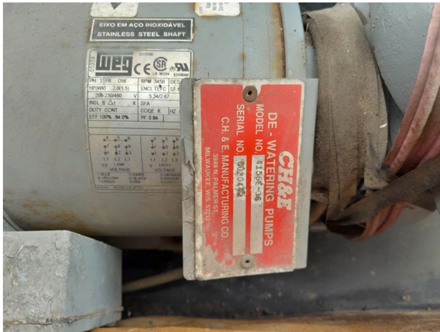
EXISTING PUMP MOTOR LABEL
