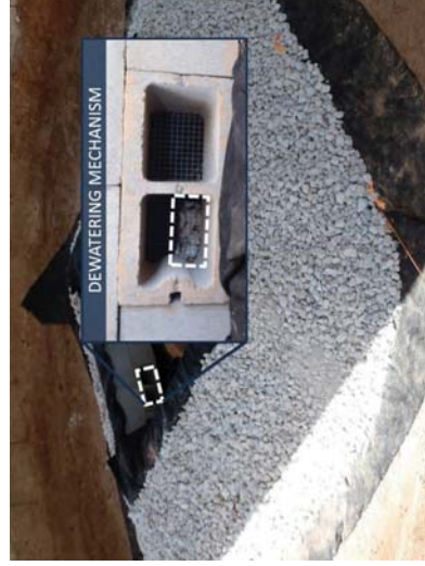
Figure IP-3 Block and Gravel Inlet Protection Installation. (Showing dewatering device.) (Photo courtesy of AU-SRF. See Appendix for CAD files)
