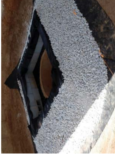
Figure IP-2 Block and Gravel Inlet Protection Installation. (Showing geotextile underlayment, gravel, and dewatering device.) (Photo courtesy of AU-SRF. See Appendix for CAD files)
