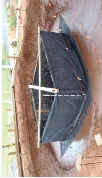
Figure IP-1 Silt Fence Inlet Protection Installation. (Showing silt fence, geotextile underlayment, steel T-posts, 2 x 4 bracing, and dewatering device.) (Photo courtesy of AU-SRF. See Appendix for CAD files)
