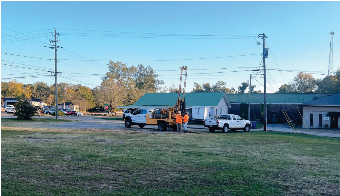
This photo is facing south across the site and shows boring B-08 in the process of being drilled.
