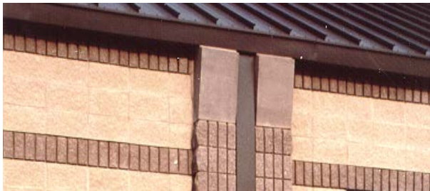
4-6c 820th SFG facility incorporates exposed gutters with downspouts recessed into pilasters.
