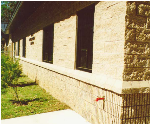
4-10a Split-face concrete masonry with special water table shape and split-rib CMU base.
