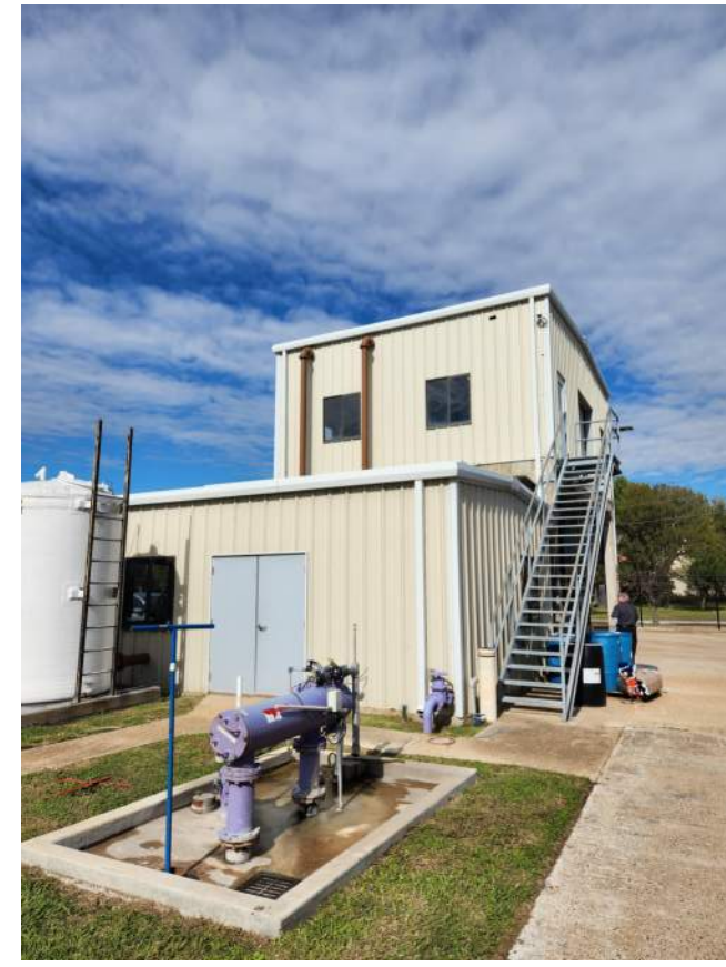
SLUDGE BELT PRESS - SOUTH
