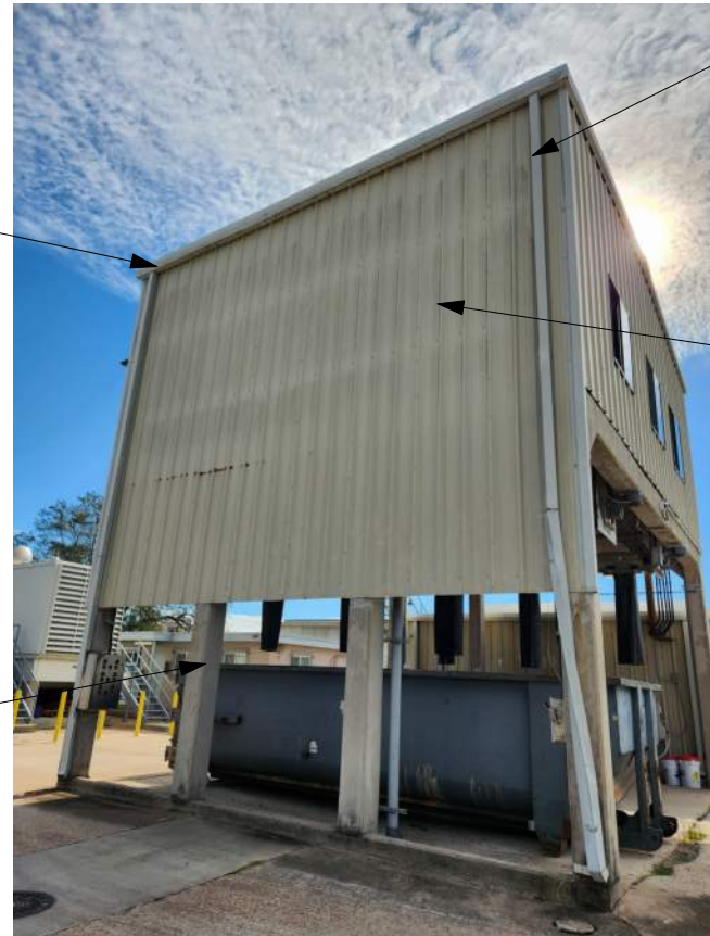
SLUDGE BELT PRESS - NORTH
