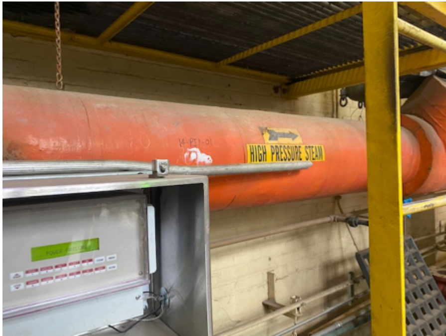
11. High Pressure Steam Pipe Insulation (HM #11)
