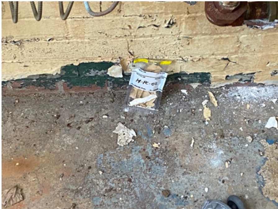
2. Beige/Yellow Paint on Brick Wall, Building 14, Boiler Room, Behind Boiler #3 (Sample #14-PC-02)
