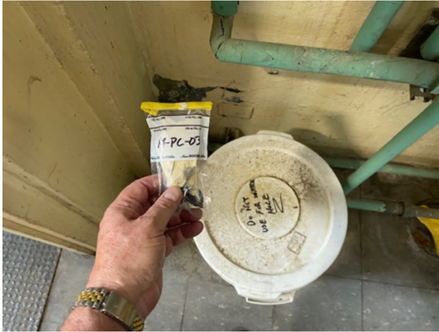
3. Beige/Yellow Paint on Concrete Wall, Building 14, Boiler Room, Front of Boiler #3 (Sample #14-PC-03)
