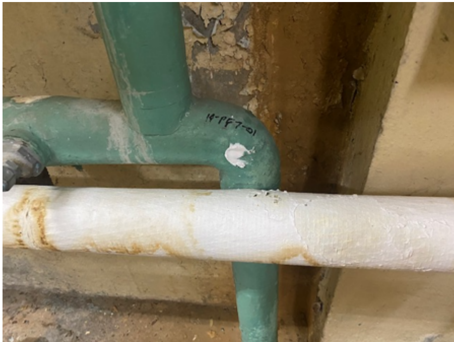
24. Hard Mudded Pipe Fitting, Cold Water (HM #24)
