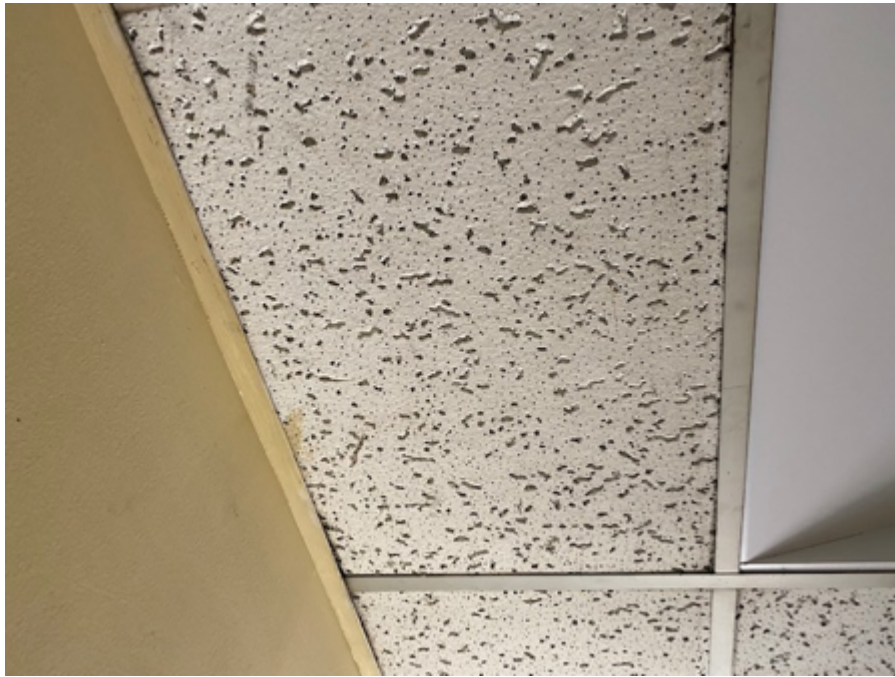
3. 2' X 2' White Ceiling Tile, Wide Fissures, Gouges and Holes (HM #3)
