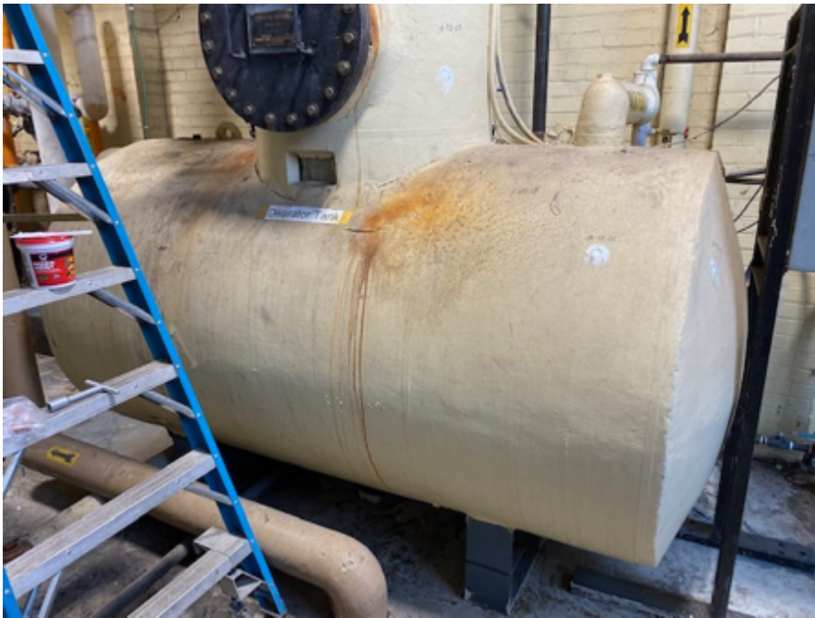
22. Deaerator Tank Insulation (HM #22)
