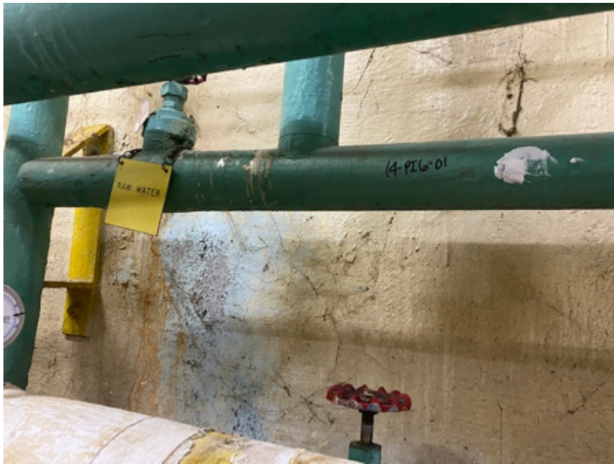
16. Raw Water Pipe Insulation, Glass Fiber Type (HM #16)
