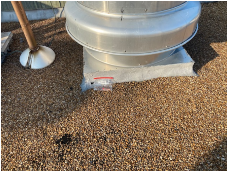
30. Silver Painted Equipment Flashing (HM #30)
