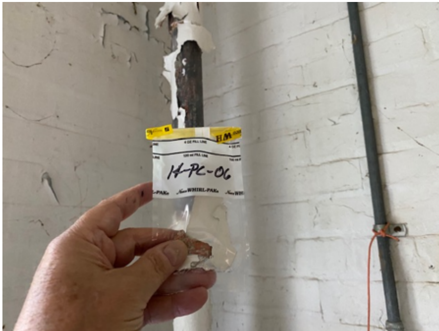
6. White Paint, Metal Conduit, Building 14, Mezzanine, Near Deaerator Tank (Sample #14-PC-06)
