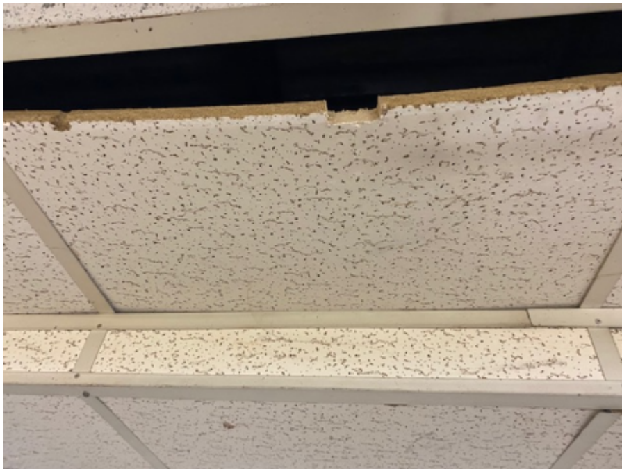
2. 2' X 2' White Ceiling Tile, Gouges and Pinholes (HM #2)
