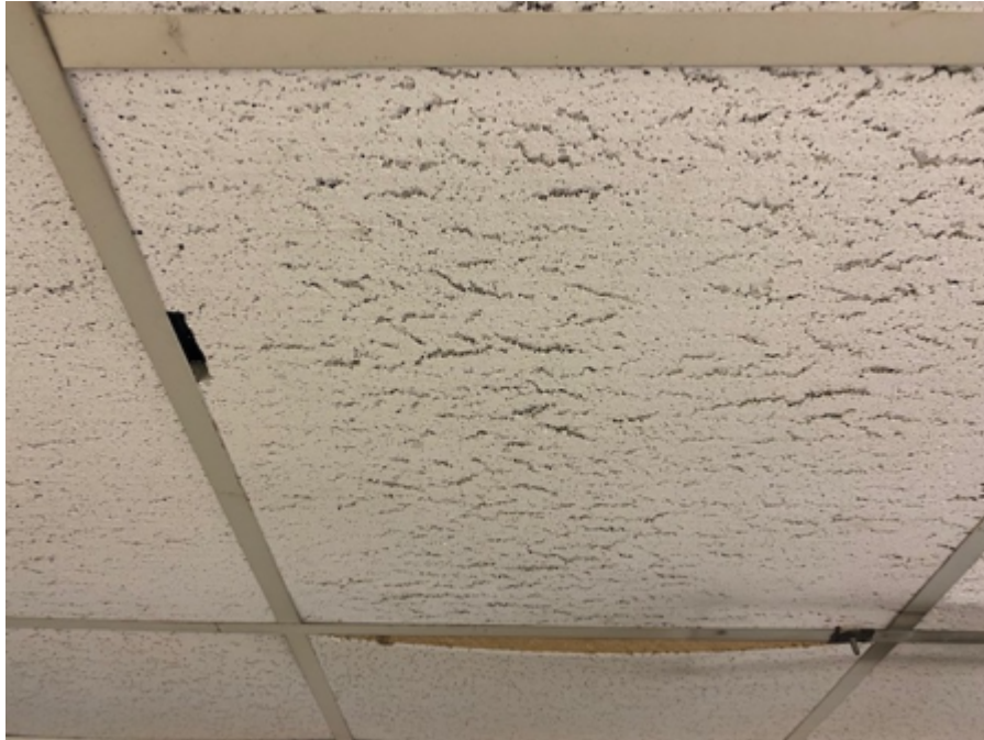
1. 2' X 2' White Ceiling Tile, Deep Fissures and Pinholes (HM #1)
