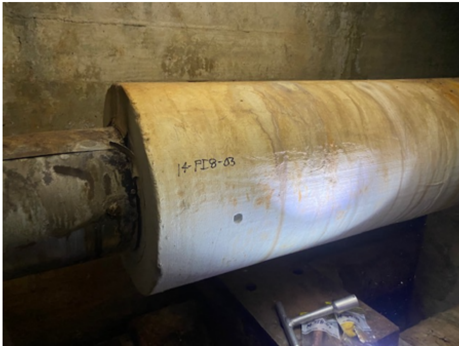
18. Medium Pressure Steam Pipe Insulation (HM #18)
