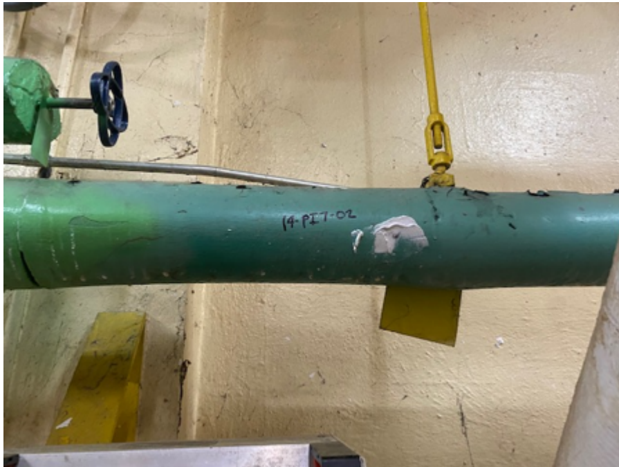
17. Cold Water Pipe Insulation (HM #17)
