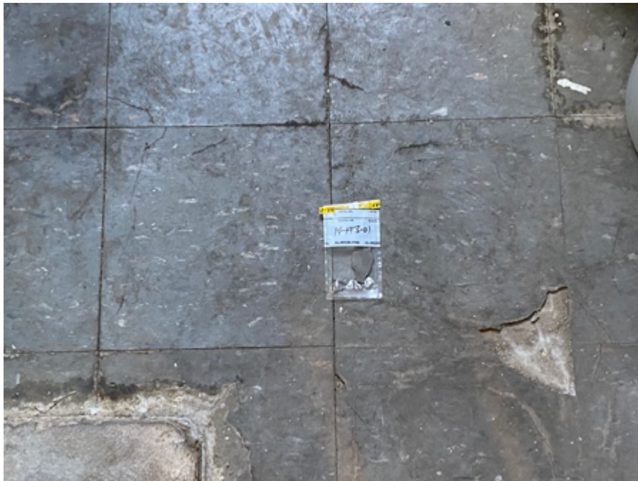
6. 12" X 12" Brown, Floor Tile and Associated Mastics, Glues & Adhesives (HM #6)
