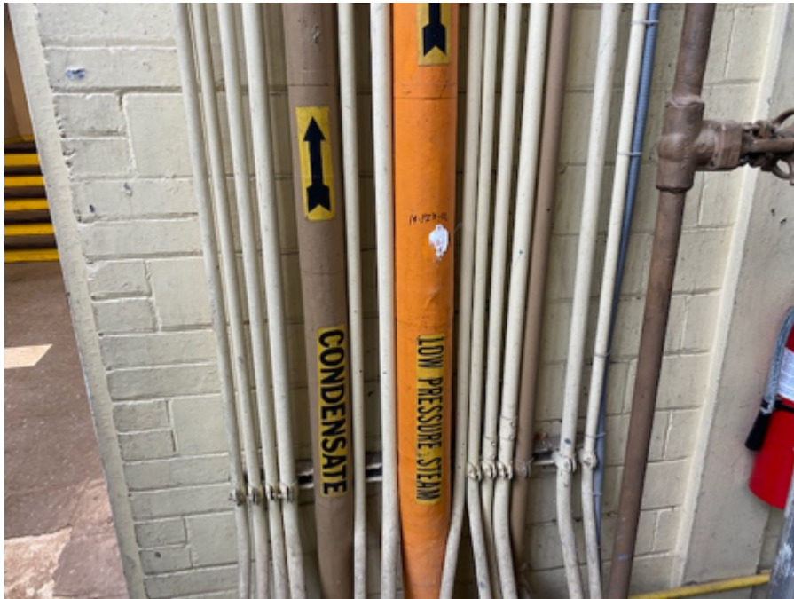
13. Low Pressure Steam Pipe Insulation (HM #13)
