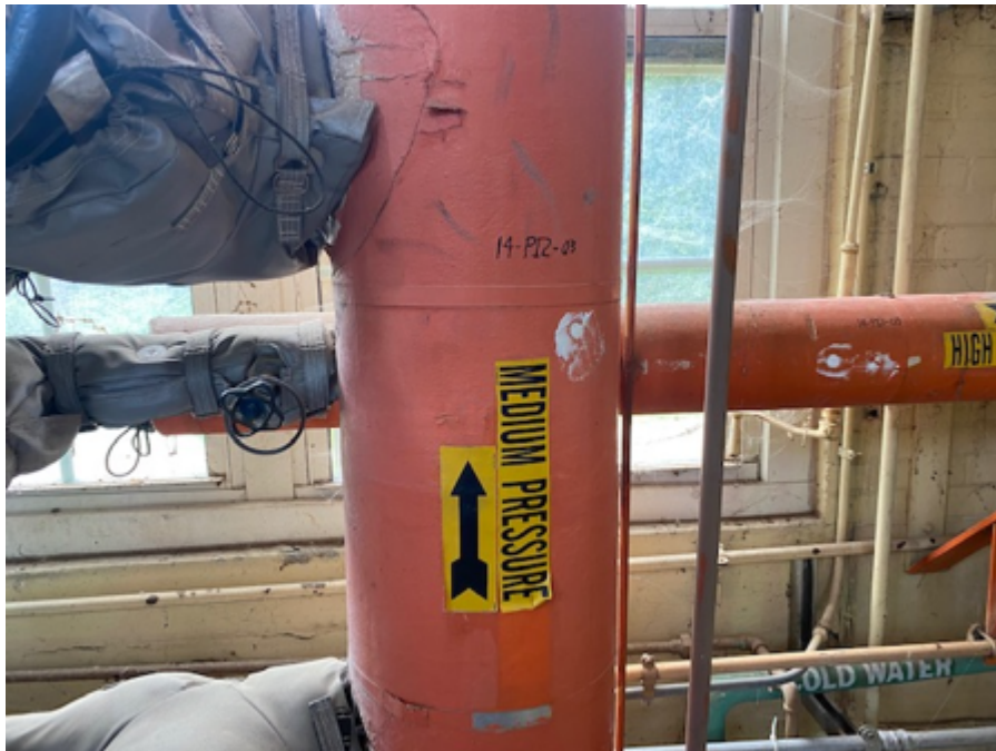
12. Medium Pressure Steam Pipe Insulation (HM #12)
