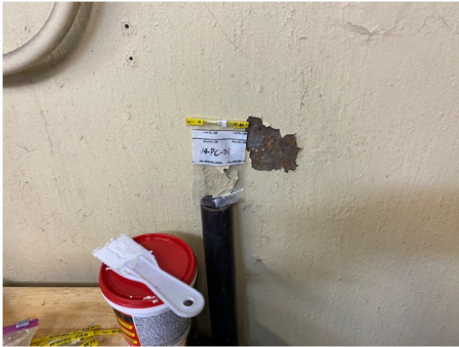
1. Beige/Yellow Paint on Concrete Wall, Building 14, Basement Shop Area (Sample #14-PC-01)
