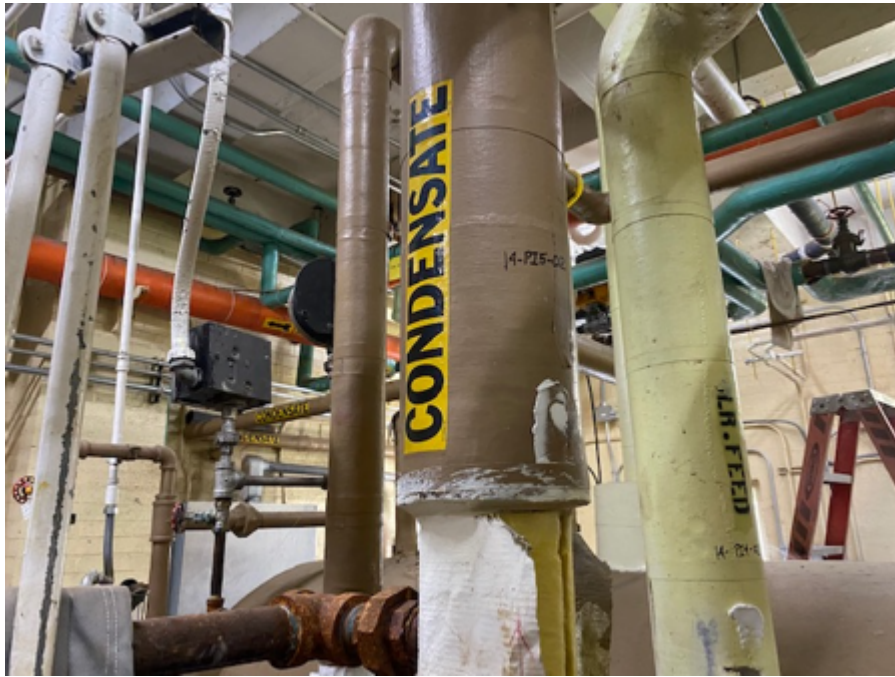
15. Condensate Pipe Insulation (HM #15)
