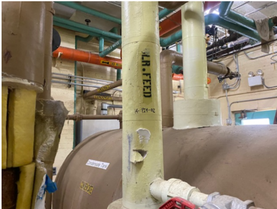
14. Boiler Feed Pipe Insulation (HM #14)
