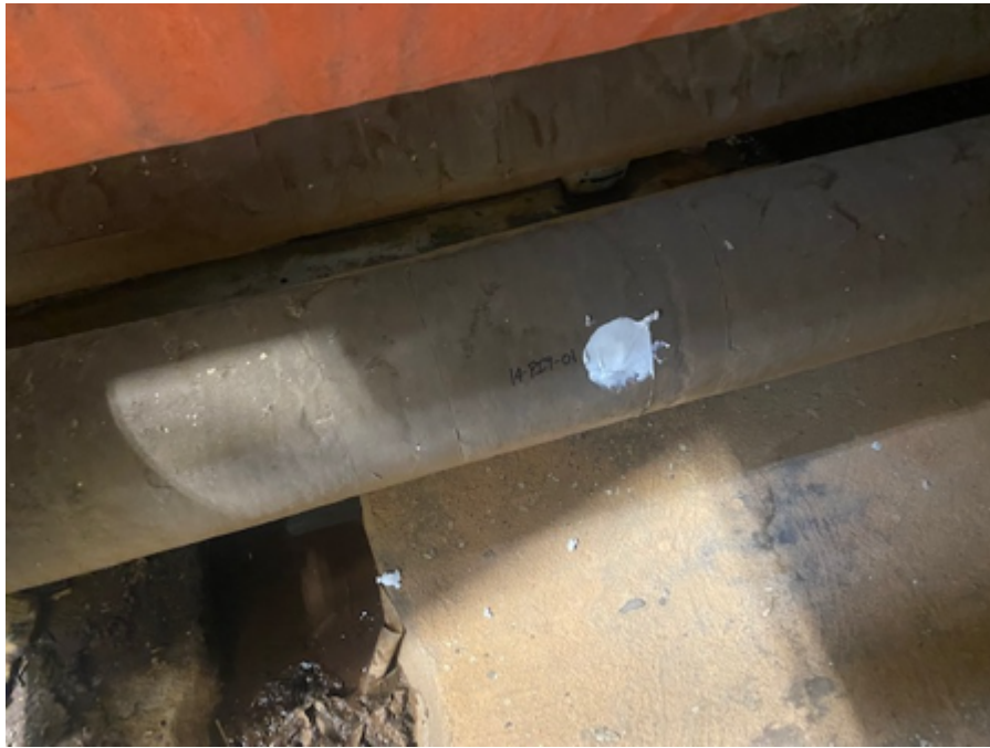
19. Condensate Return Pipe Insulation (HM #19)
