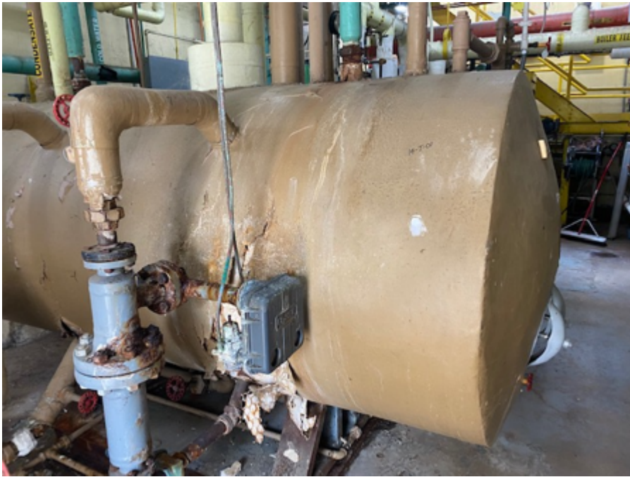
21. Condensate Tank Insulation (HM #21)
