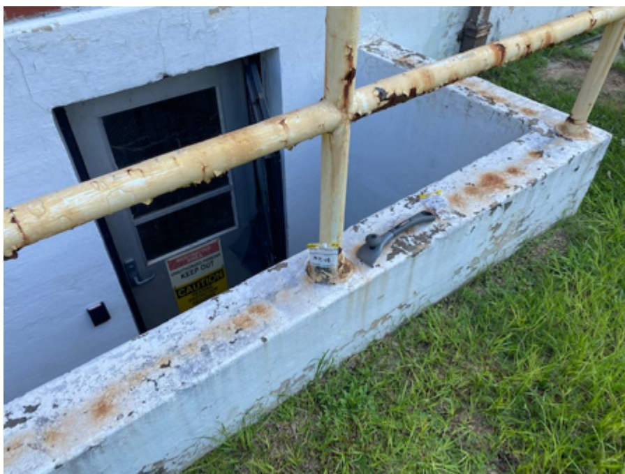
8. Yellow Paint on Exterior Metal Stair Rail, Building 14, Exterior (Sample #14-PC-08)
