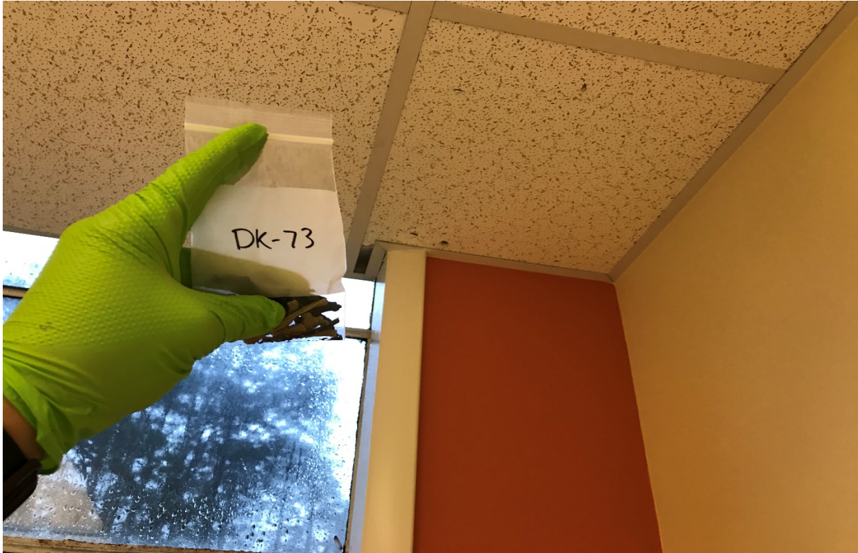
Plate 6: Laboratory analyses detected 5% chrysotile asbestos minerals within the black mastic of samples DK-70, DK-73, and DK-75 collected from behind the drywall above the drop ceiling of the large veterinarian office patient room.
