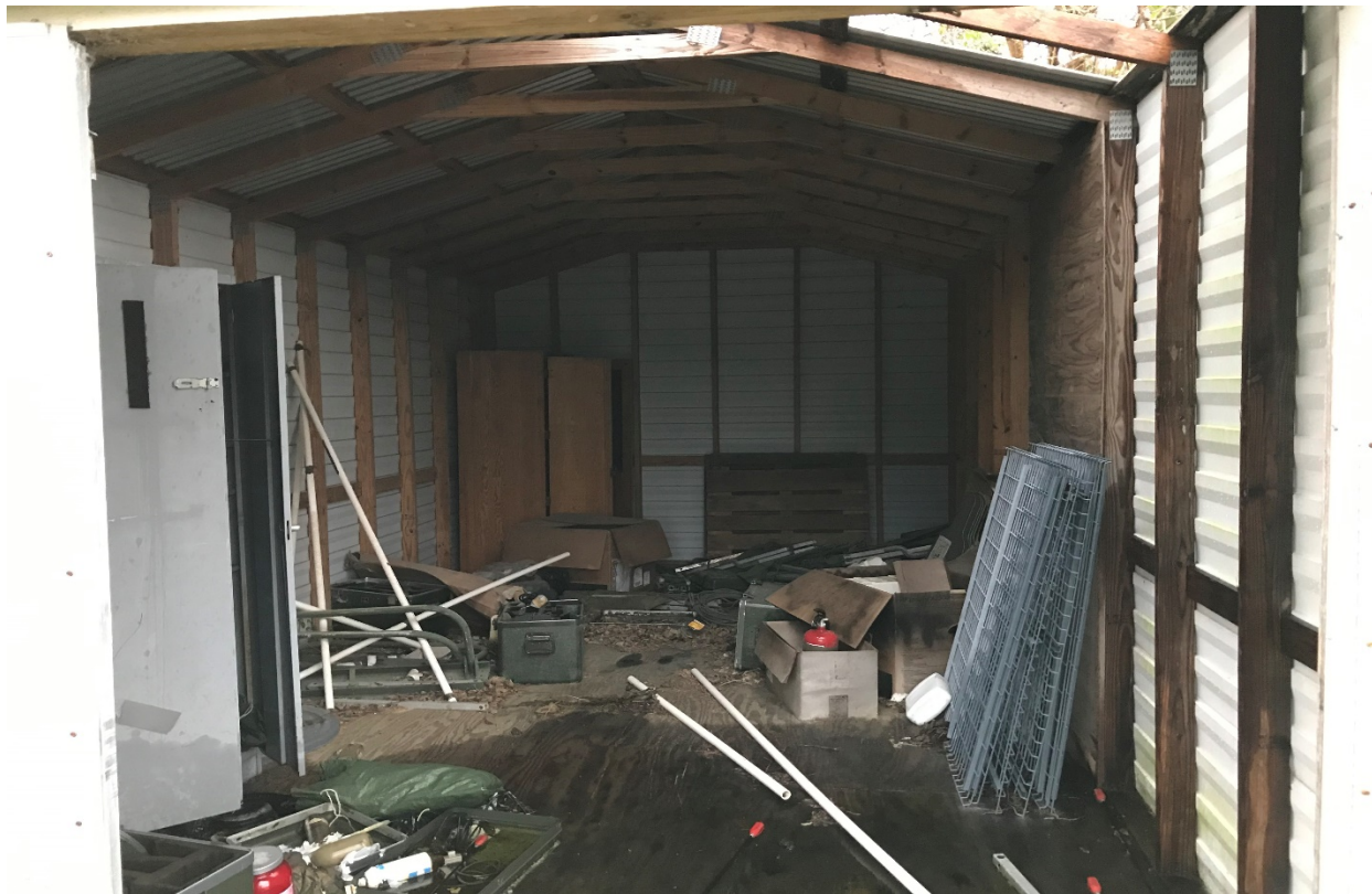
Plate 4: Interior of one of the metal sheds with large damage observed to the exterior.
