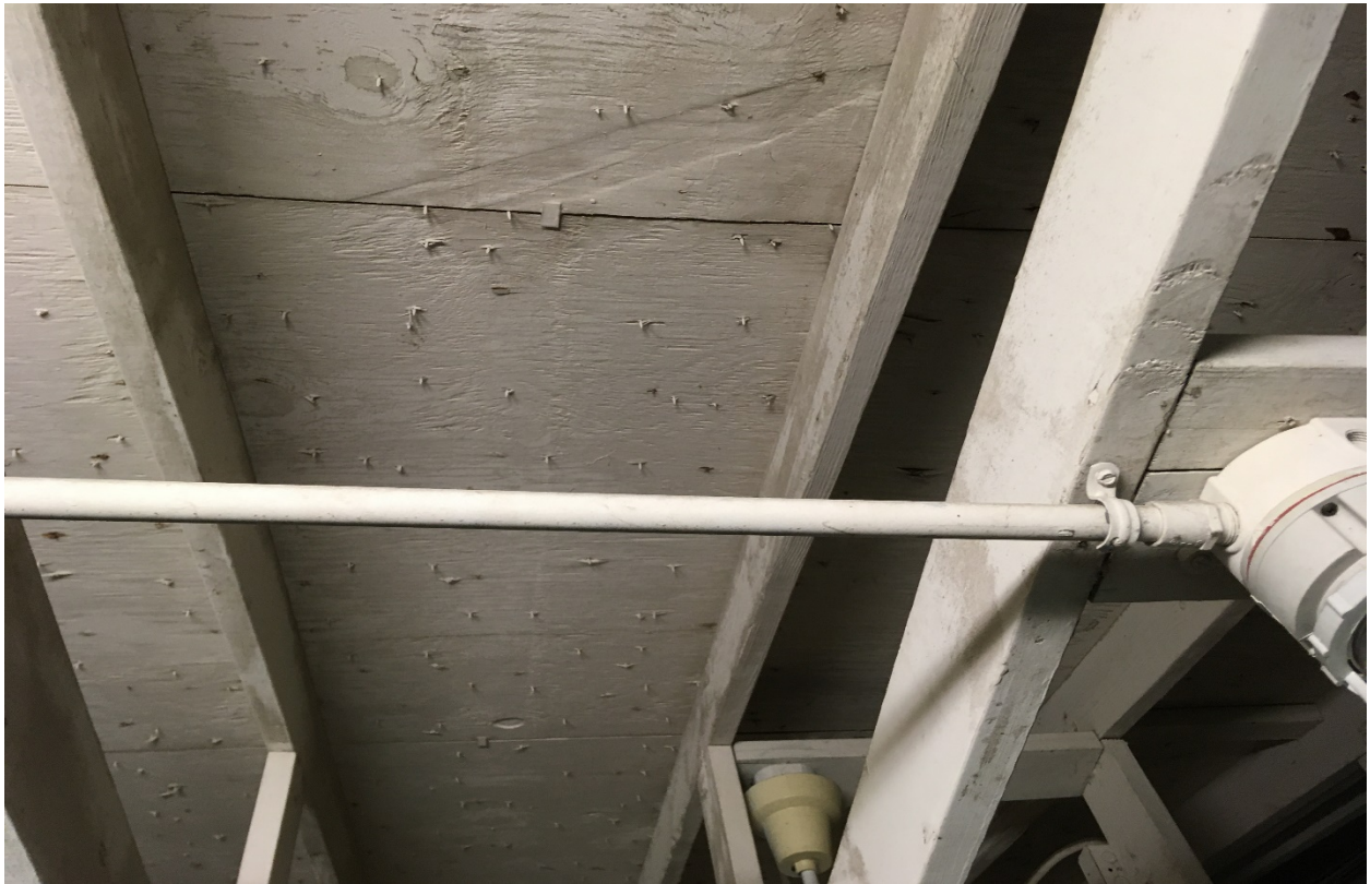
Plate 10: During time of site visit the underside of the roof appeared to have nail penetrations indicative of an asphalt shingle roof.
