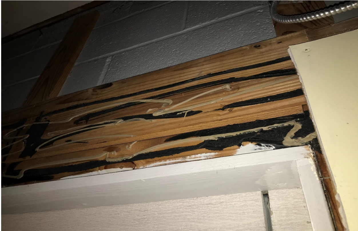
Plate 8: Samples DK-70, DK-73, and DK-75 were collected from behind the drywall above the drop ceiling of the large veterinarian office patient room. The sample locations are represented by the picture above.
