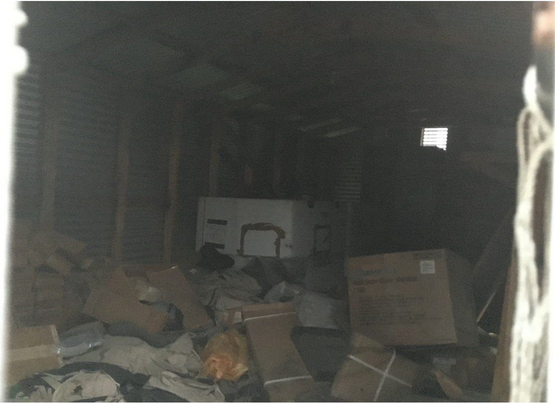
Plate 3: Interior of one of the metal sheds with less damage observed to the exterior.
